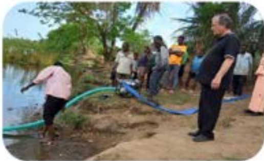
Delivered and now testing one of the water pumps in Chikwawa district
